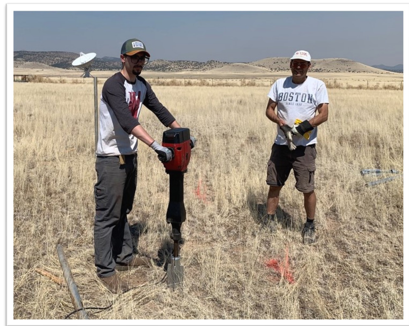
Prof Taylor and I installing antenna masts using a jackhammer at the LWA-NA site
