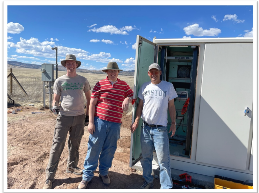
Electronics Shelter Installation on-site (+Pratik)
